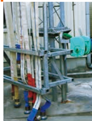
For drying a fire-fighting hose
